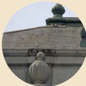
Inappropriate building material
